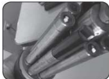
Figure 5 - Wiped C/T sensor in optimal position ready to be secured
